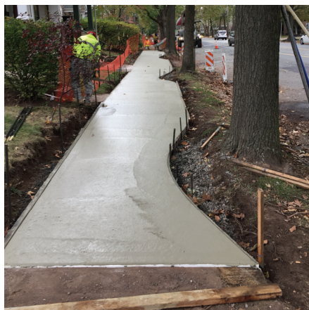
NEW SIDEWALK is installed last November on the 1100 block of High Street. More than 15,000 square feet of sidewalks were replaced with federal Walk/Bike Pottstown grant money.
