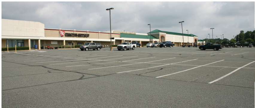
MASSIVE RUNOFF — Huge parking lots like this one at Pottstown Plaza on State Street cause an enormous amount of stormwater runoff that must be mitigated before it causes flooding and the pollution of our waterways. Stormwater will cost millions of dollars to manage.
